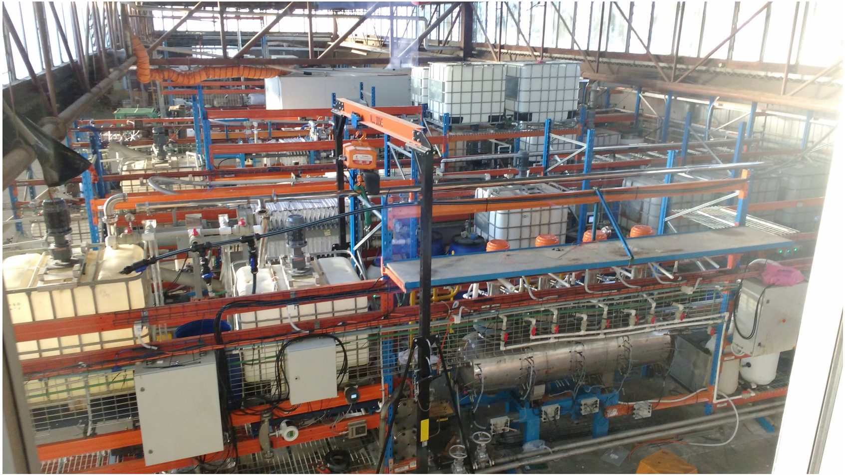
Photo of the fully-completed demonstrated-scale processing plant constructed on Simulus Engineering's premises in Perth, Australia that which is presently delivery battery metals (cobalt sulphate and nickel sulphate) to SK Innovations
